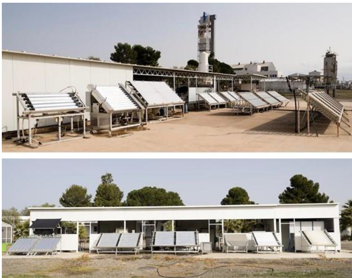
Figure 86. View of several CPC photo-reactors for purification of water. water (up) CPC facilities I (down) CPC facilities II.
