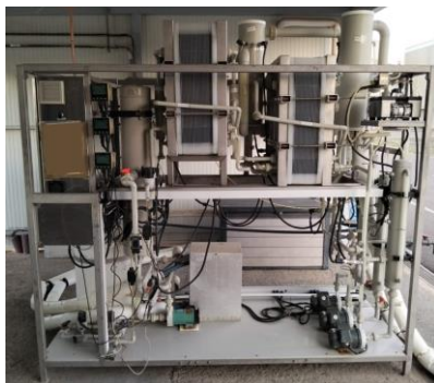
Figure 80. The FVMED plant installed at CIEMAT-PSA.
