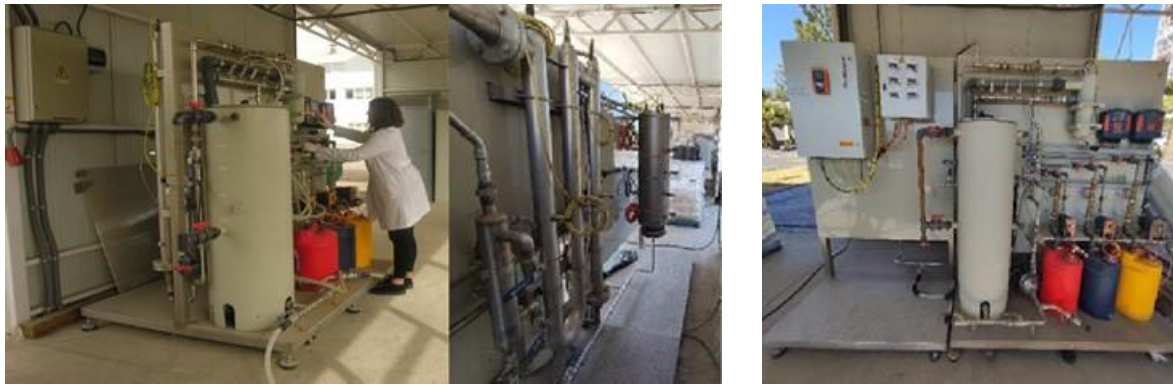
Figure 91. UVC pilot plant installed at PSA facilities (left) and recent improvements (right).
