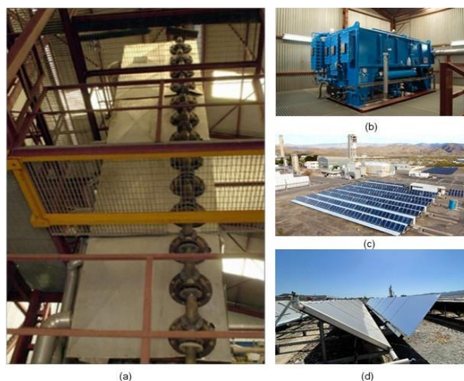
Figure 79. The PSA SOL-14 MED Plant (a) double-effect LiBr-H 2 O absorption heat pump (b) and 606-m 2 flat plate solar collector field with tracking mirrors (c and d).
