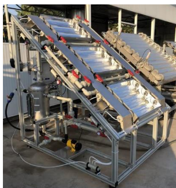
Figure 95. Solar CPC with direct injection of ozone available at PSA facilities
