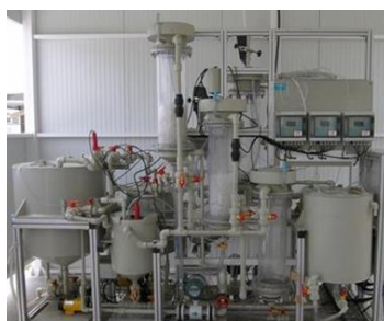
Figure 101. Biological pilot plant installed at PSA facilities.
