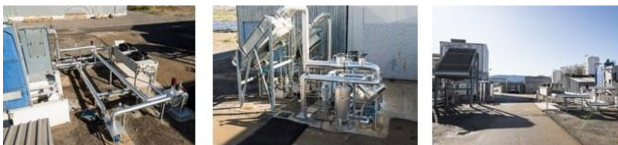
Figure 85. The PSA Cooling Facility. a) Wet Cooling tower and Air Cooled Heat Exchanger (Innovative Combined Cooling System); b) Steam generator connected to the Air Cooled Condenser and to the Surface Condenser; c) General view of the Cooling Facility
