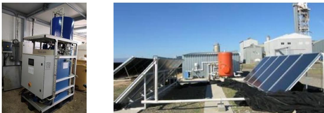
Figure 81. Internal (Left) and external (right) views of the Membrane Distillation experimental test bed within the PSA low-temperature solar thermal desalination facility.
